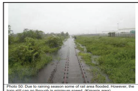
Photo 50: Due to raining season some of rail area flooded. However, the train still can go through in minimum speed. (Kimanis area)
