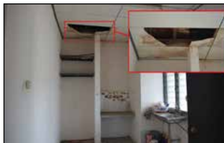
Unit G005, Kwarters DCA Langkawi - Siling Dapur Pecah (23.07.2014)
