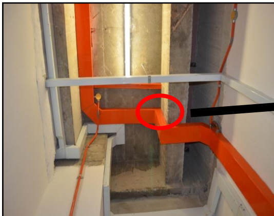
GAMBAR 15.7 Tiada Copper Bridge Dipasang Di Sambungan Trunking
