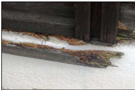
12 Rejimen Askar Melayu Di Raja Kem Daralockwood, Kuantan - Keadaan Dinding Reput Di Berek Bujang
