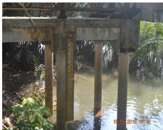
Gambar 1.5 Stesen Aras Air
