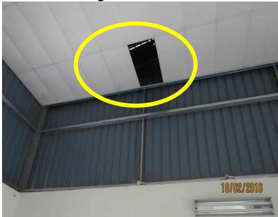
Gambar 4.23 Siling Asbestos Pecah
