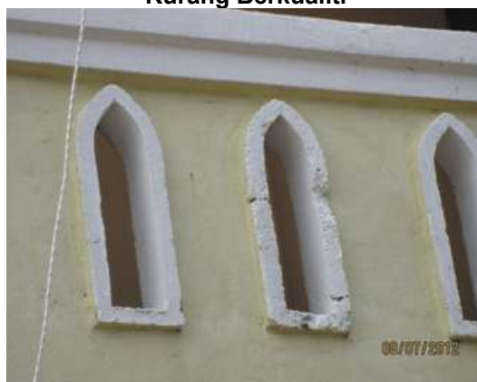
Gambar 3.24 Kemasan Decorative Precast Concrete Kurang Berkualiti
