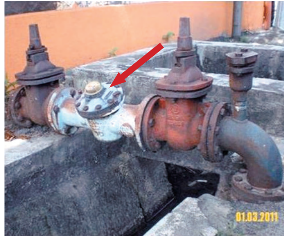
Gambar 8.7 Bulk Meter Rosak
