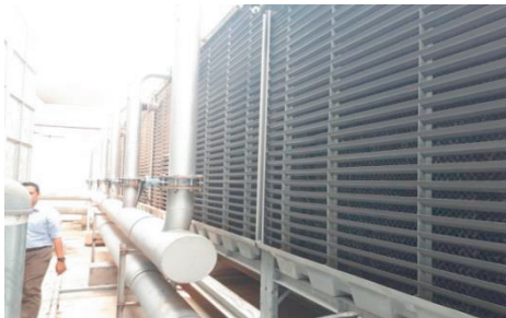
Loji Cooling Tower
