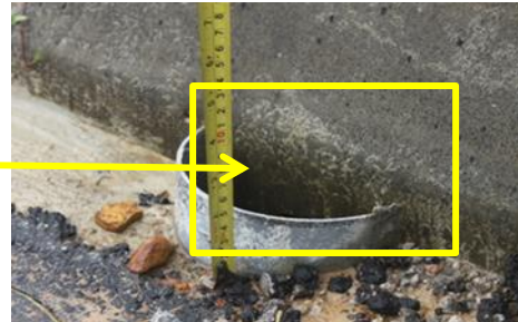
CH3275 Phase 5 Stage 1 - Proposed Samalaju Boulevard Package 1 - Aras Saliran Masuk (Inlet Scupper Drain) Tinggi Daripada Aras Jalan (03.10.2018)
