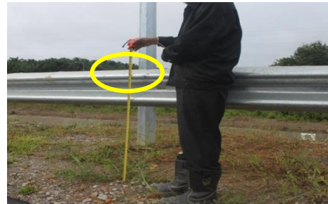
CH3200 Phase 5 Stage 1- Proposed Samalaju Boulevard Package 1 - Guardrail Dipasang Tinggi Daripada Lukisan (03.10.2018)
