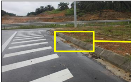
CH3275 Phase 5 Stage 1 - Proposed Samalaju Boulevard Package 1 - Aras Saliran Masuk (Inlet Scupper Drain) Tinggi Daripada Aras Jalan (03.10.2018)
