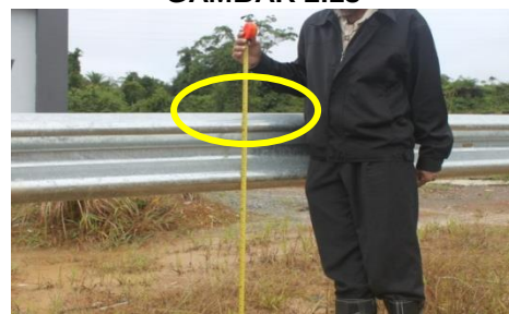
CH2800 Phase 5 Stage 1- Proposed Samalaju Boulevard Package 1 - Guardrail Dipasang Tinggi Daripada Lukisan (03.10.2018)
