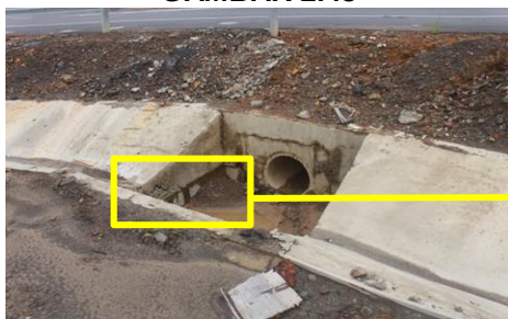
CH3200 Persimpangan B1 (Phase 5 Stage 1- Proposed Samalaju Boulevard Package 1) - Honeycomb pada Kawasan Outlet Outfall Drain (03.10.2018)
