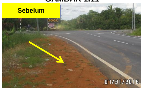
Jambatan Batang Samarahan ( Road Widening to Connect Jalan Muara Tuang/Semera/Pendam Junction ) - Spot Turfing Tidak Ditanam di Sebahagian Bahu Jalan (31.07.2018)
