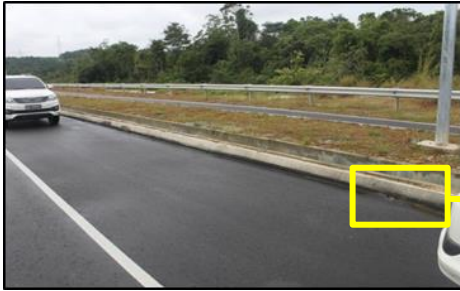
CH2750-CH2850 Phase 5 Stage 1 - Proposed Samalaju Boulevard Package 1 - Saliran Masuk (Inlet Scupper Drain) Tersumbat dan Tertutup (03.10.2018)
