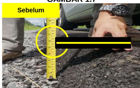
Jambatan Batang Samarahan (Road Widening To Connect Jalan Muara Tuang/Semera/Pendam Junction) - Bahu Jalan ( Unpaved Shoulder ) Rendah Daripada Permukaan Pavement (31.07.2018)
