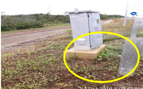
Distribution Pillar No.1 Phase 5 Stage 1 - Proposed Samalaju Boulevard Package 1 - Kotak Pbumian (Earthing Chamber) Tidak Ditemui Berhampiran Distribution Pillar (03.10.2018)
