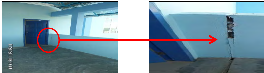
Phase 2 Package 1 Bahagian Mukah, Sarawak - Expansion Joint Retak (20.07.2017)
