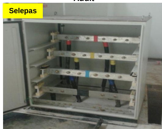
Gambar 2.8 Cables Are Terminated In The Rental Genset Interface Board Selepas Teguran Audit
