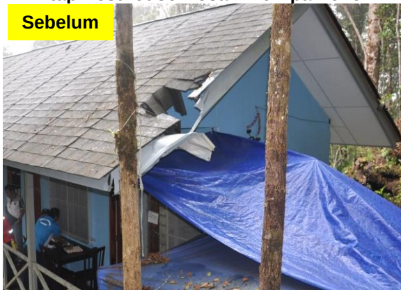
Gambar 7.39 Atap Resthouse Rosak Ditimpa Pokok
