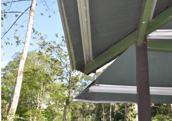
Gambar 7.41 Atap Timber Cover Deck Rosak Ditimpa Kayu
