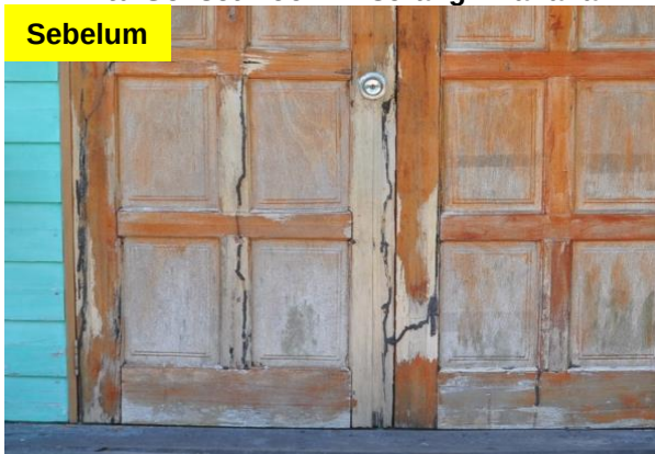
Gambar 7.33 Pintu Genset Room Diserang Anai-anai
