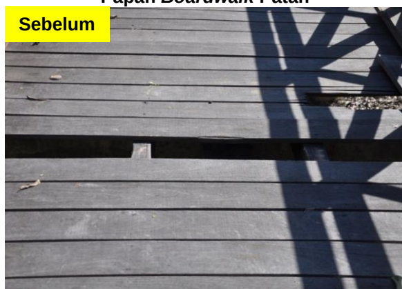
Gambar 7.25 Papan Boardwalk Patah
