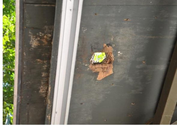
Gambar 7.42 Atap Timber Cover Deck Rosak Ditembusi Kayu
