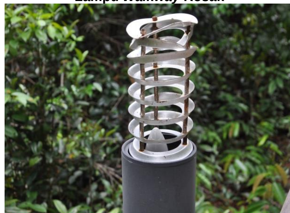
Gambar 7.52 Lampu Walkway Rosak
