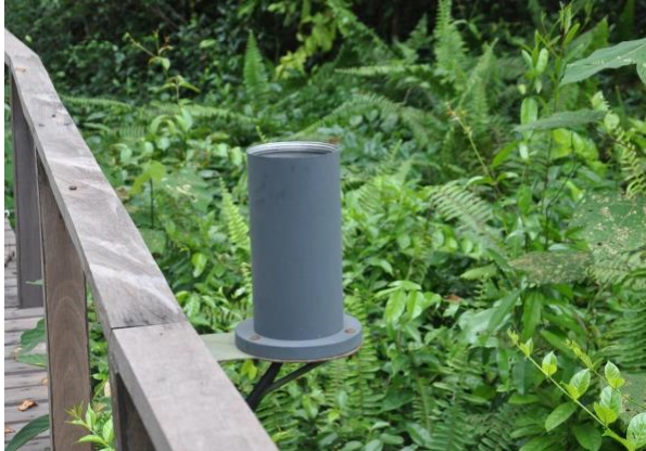
Gambar 7.53 Lampu Walkway Rosak
