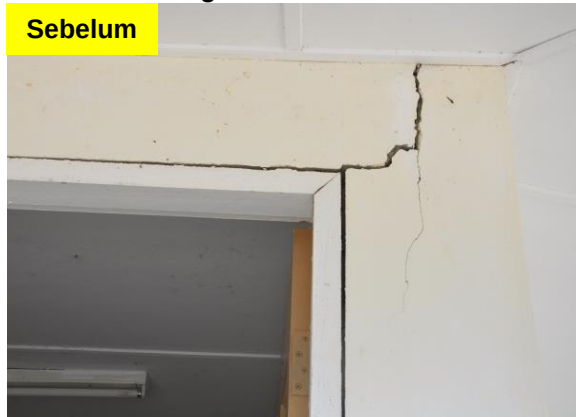
Gambar 7.35 Dinding Guard House Retak
