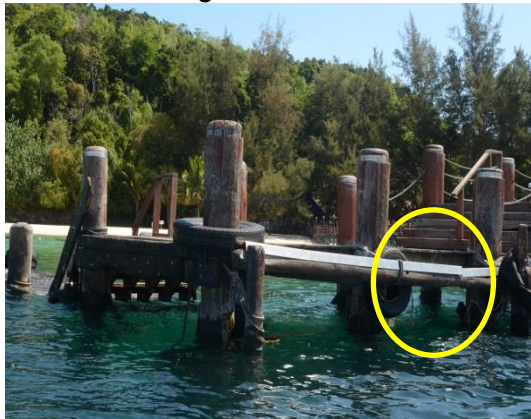
Gambar 5.15 Tiang Fender Rosak
