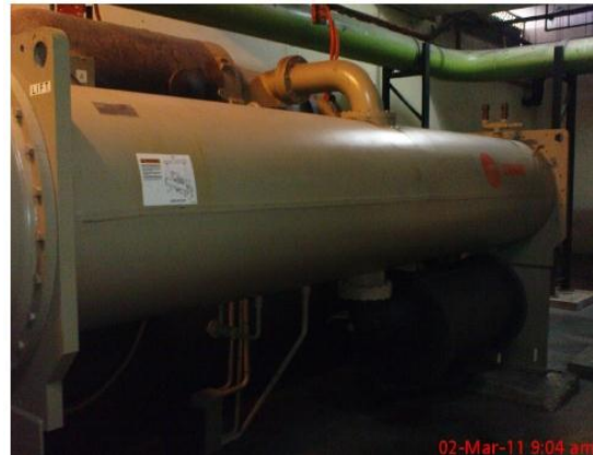
Gambar 6.4 Chiller Auto Trans 3.3kv Rosak
