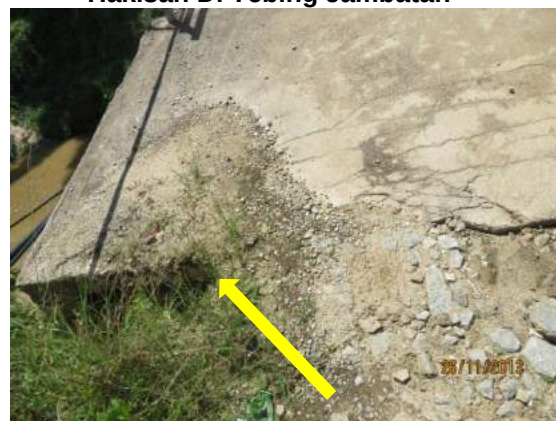
Gambar 4.14 Hakisan Di Tebing Jambatan
