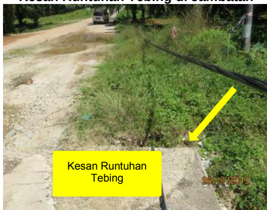
Gambar 4.13 Kesan Runtuhan Tebing di Jambatan
