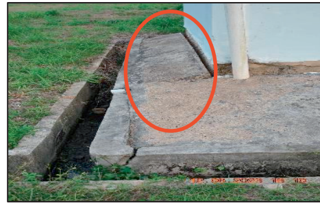
Air Blower Room
