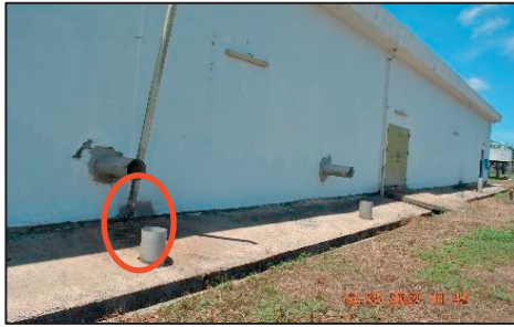
Air Blower Room
