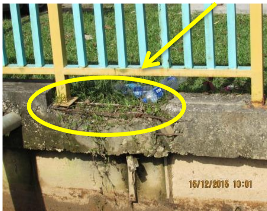
Gambar 2.15 Capping Beam Pecah
