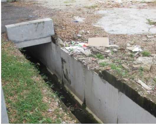
Gambar 2.16 Capping Beam Pecah
