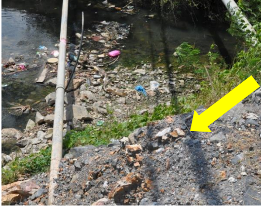
Gambar 1.21 Hakisan Tebing Bahu Jalan
