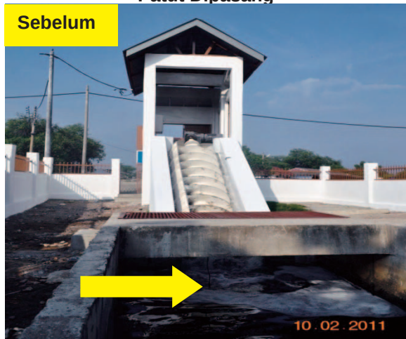
Gambar 4.10 Lokasi Aluminium Trash Screen Patut Dipasang
