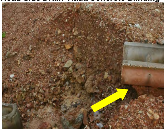
Gambar 5.15 Road Side Drain Tiada Concrete Blinding
