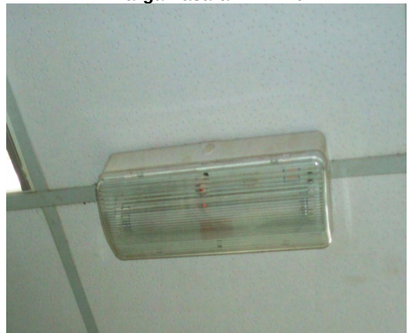
Gambar 11.13 Emergency Light c/w 3 Hrs Back-up Battery Dibayar RM200 Berbanding Harga Pasaran RM110
